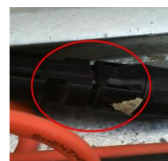
The cable is loose
