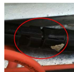
The cable is loose
